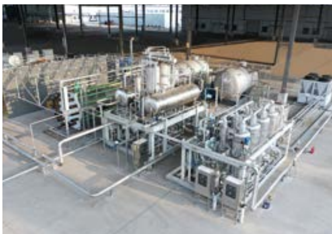
Alkaline Water Electrolytic (AWE) Hydrogen Production System
